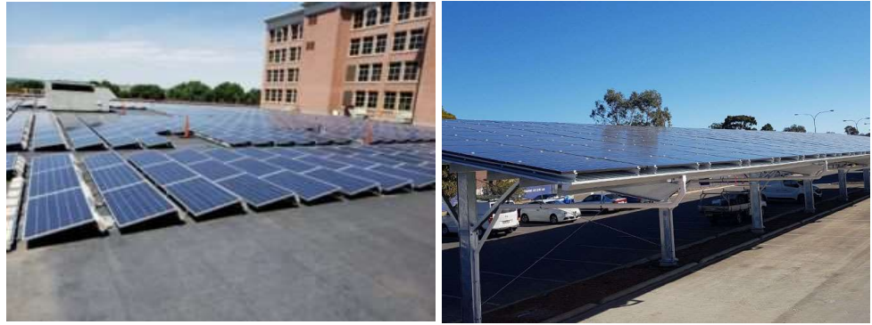
Figure 2. Example of Fixed-tilt Rooftop and Carport Solar PV Arrays
