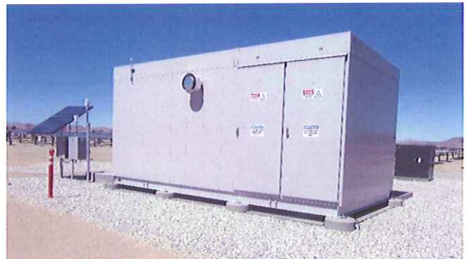
Figure 5. Typical Solar Field Switchgear
