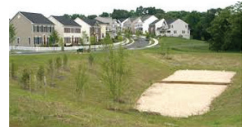
Sand filter at the base of the bioswale promotes infiltration.
