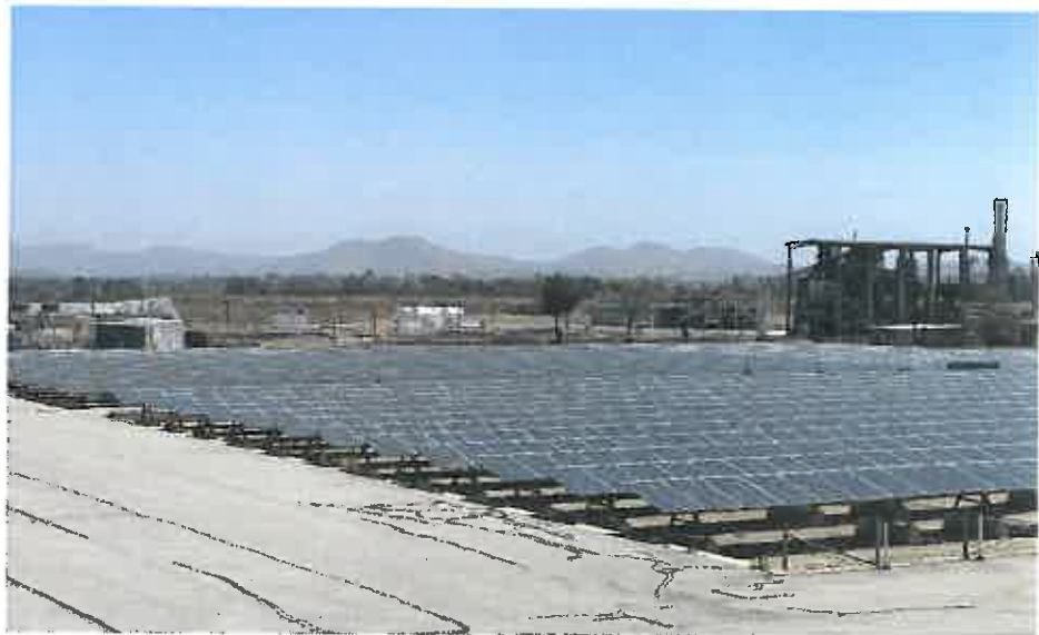
Corona's resources include wholesale solar and a solar facility at Water Reclamation Plant 1.
