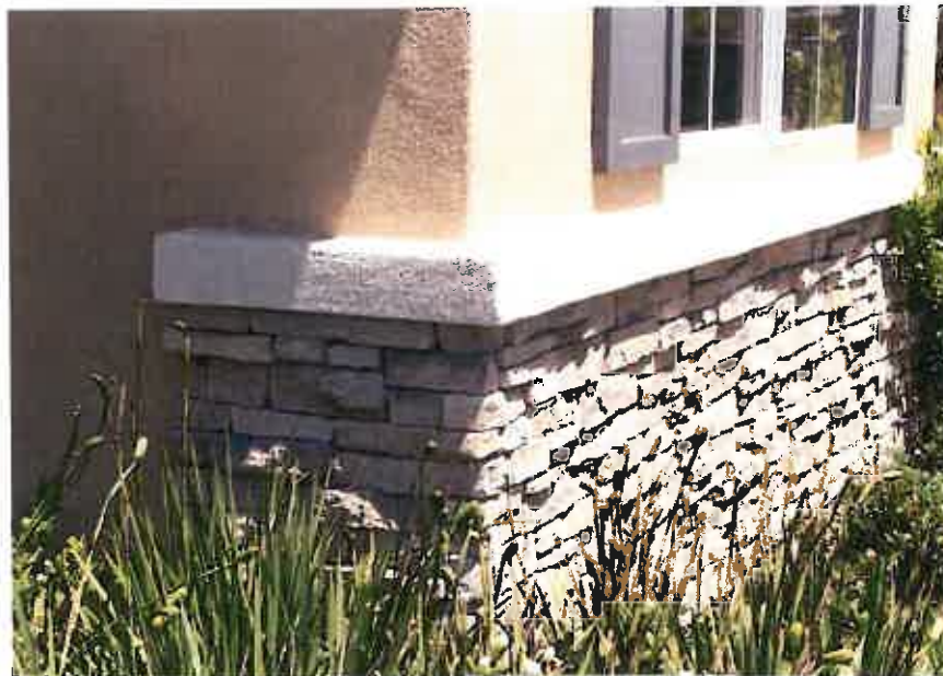
Accent material should wrap the corner of a building façade and end in a clean manner. This example displays a clean and simple top band detail that is used as a material break between the foundation accent material and the primary stucco finish.
