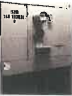
LINE SIDE CONNECTION PHOTO
